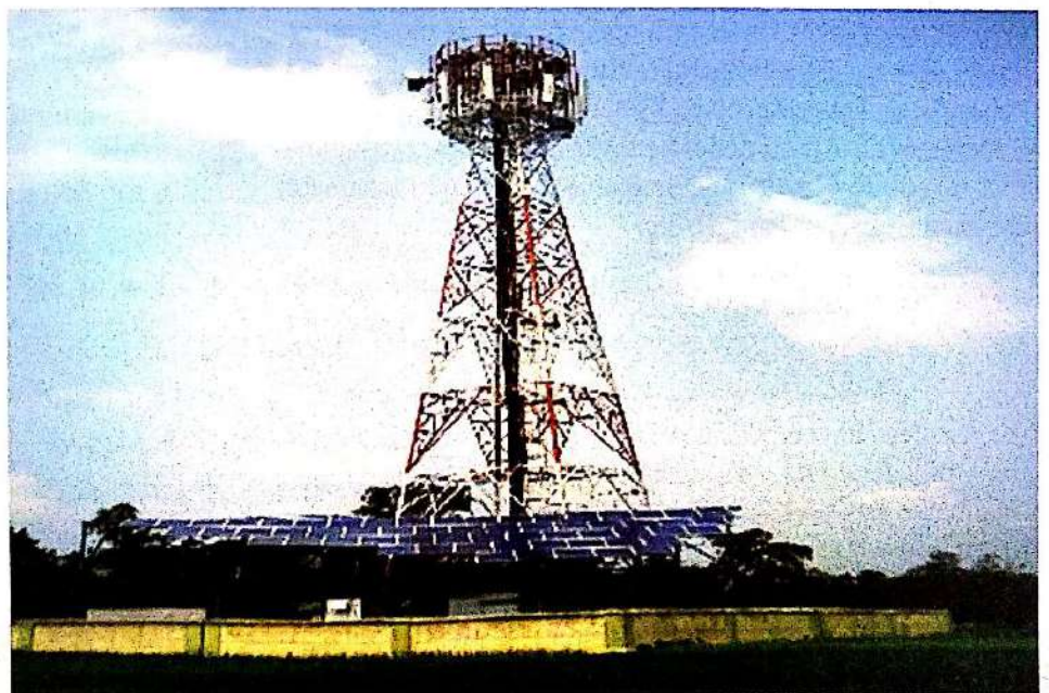
Hybrid power supply to telecom towers
